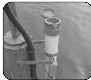
Mounted to Pier
